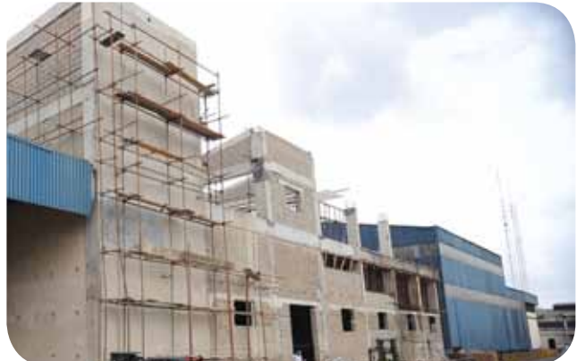
Six (6) additional sachet lines will be installed at the Powder Factory to meet increasing demand for our premium powder products. However, to accommodate these new sachet lines, a new building is being constructed.
