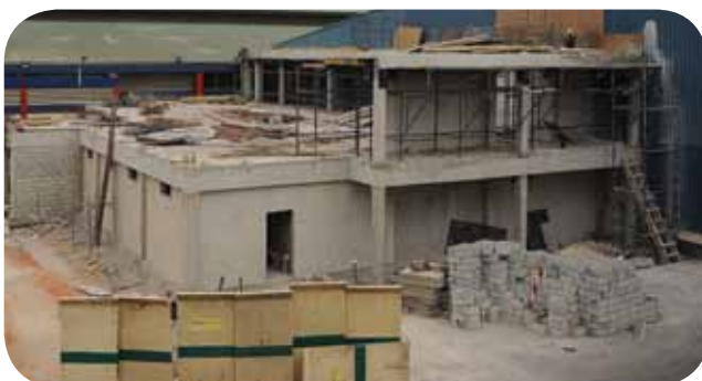
A hygiene junction is under construction for the Evaporated Milk Factory; this will ensure high level of hygiene in the factory.
