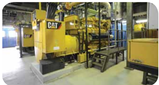
With the increased instability in the supply of Natural Gas in the country, a gas engine-driven generator has been procured to minimize the heavy costs of maintaining diesel-powered generators used in the Independent Power Plant (IPP).
