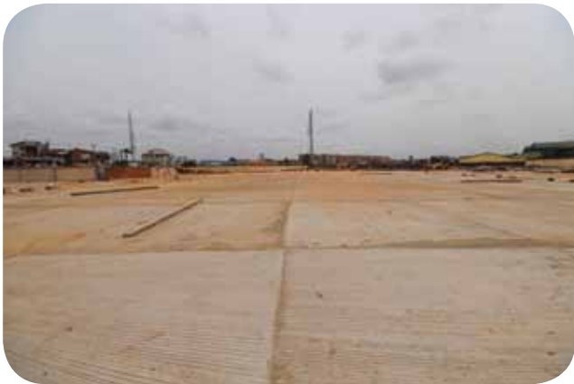
A new car park for staff is under construction in line with the master plan of the factory.
