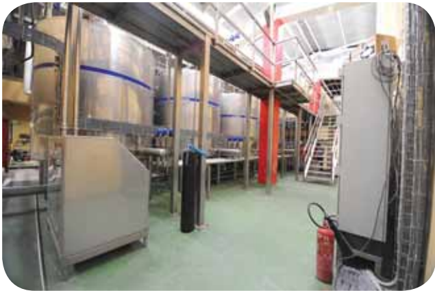
New CIP (Cleaning in Progress) kitchen has been installed at the Evaporated Milk Factory to cater for the growing demand of Evap. This newly installed CIP kitchen will boost efficiency by cleaning multiple objects per time, thereby reducing waiting time.
