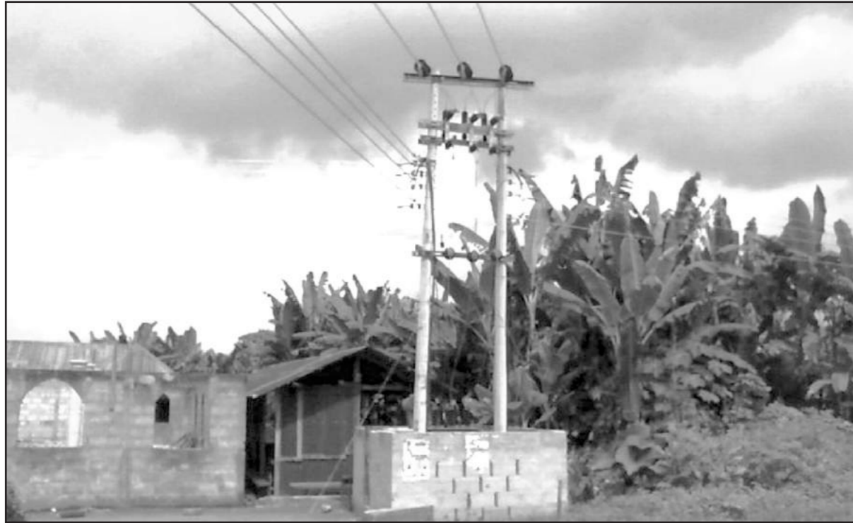
Power stepdown transformer station at Oshiugbokor Community
