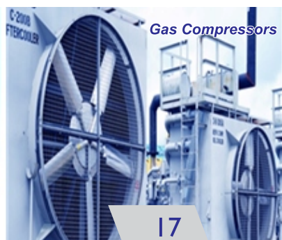
Ogbele Gas Plant and Flare Stack
