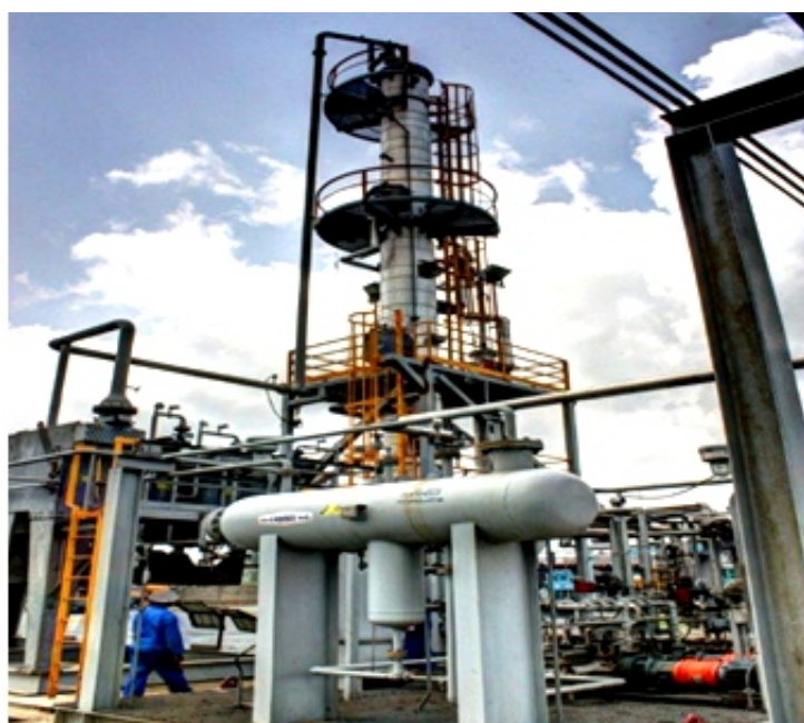
Ogbele Mini Refinery (Diesel Topping Plant)
